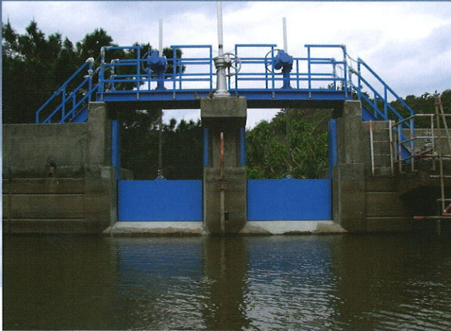
Hydraulic gate • Operation bridge
