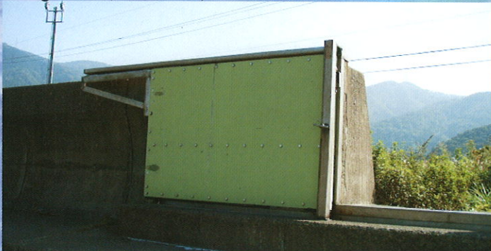
Tide barrier gate (horizontal sliding type)
